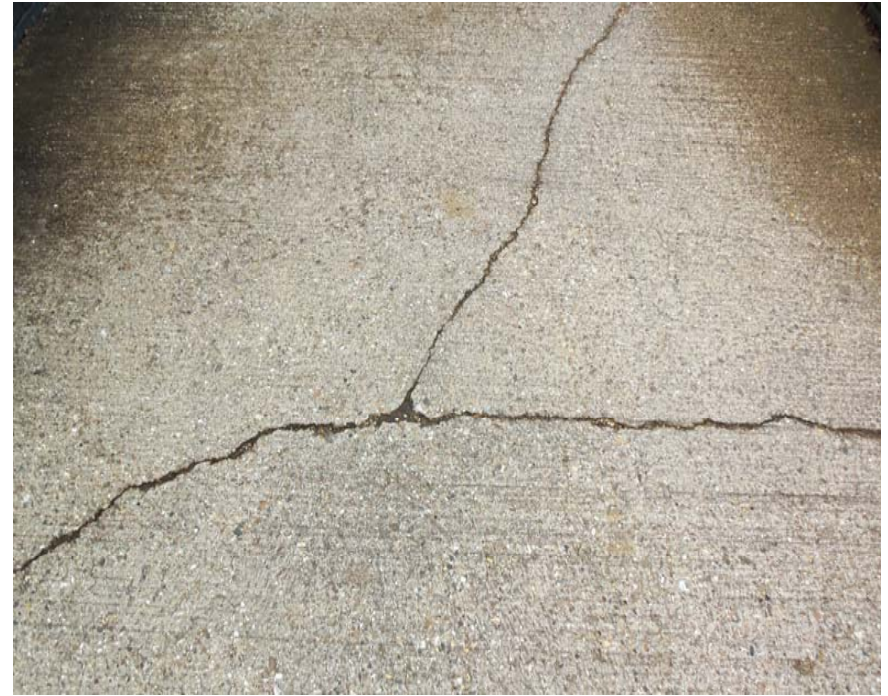
Diagonal cracks caused by settlement of the basecourse, requiring full slab replacement
