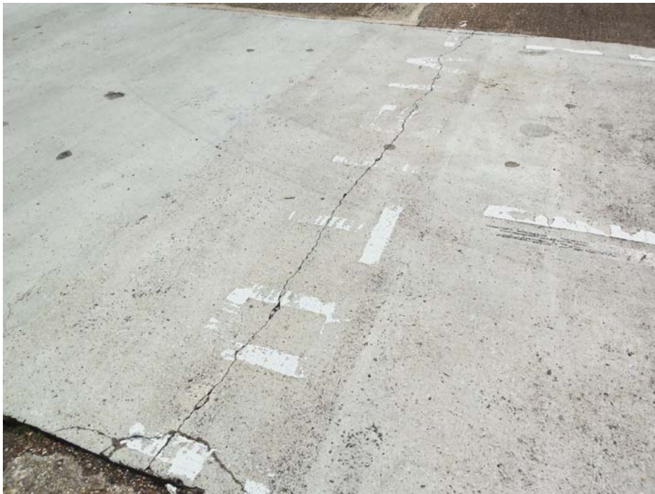
Transverse crack caused by slab flexure, requiring grout injection, resin injection or dowelling
