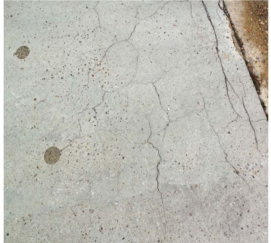
Surface crazing : poor curing
