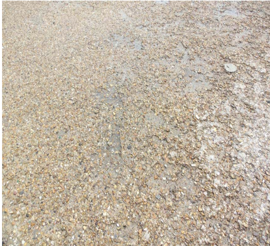
Surface erosion due to frost
